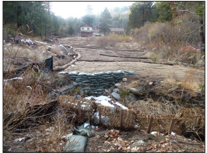
Erosion from recent rain storm at the Serenity Conference Center
