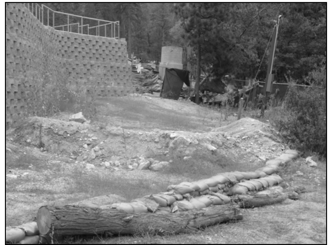
Wall and disintegrating sand bags at Eagle Ridge site.
